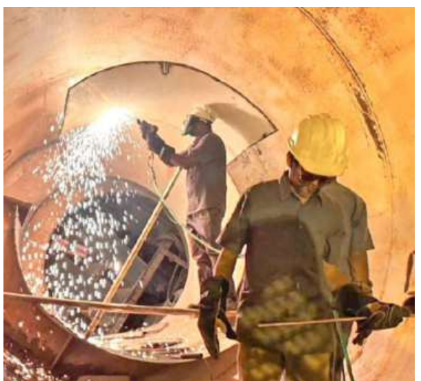
Tough task: Rescue operation under way to trace the workers trapped inside the partially collapsed SLBC tunnel on Saturday. PTI
